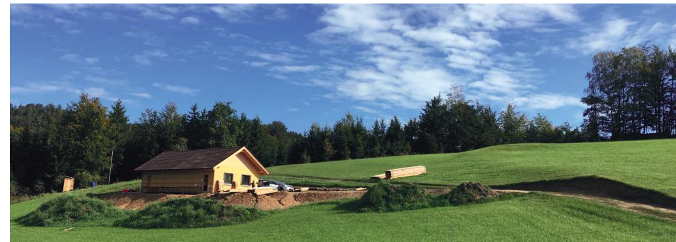
The temporary meditation hall. To the right of it and above one sees the construction site for the centre buildings.
